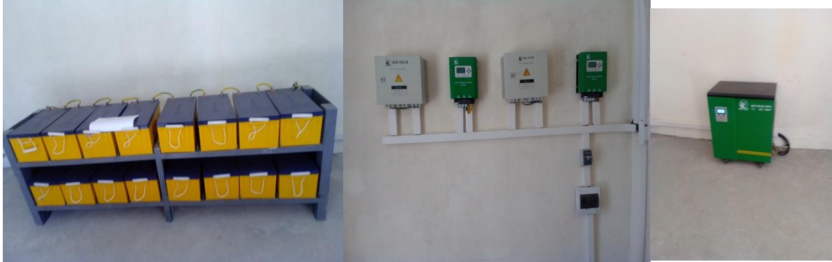
Figure 13: The all-inclusive 10 Kw Solar Power System
